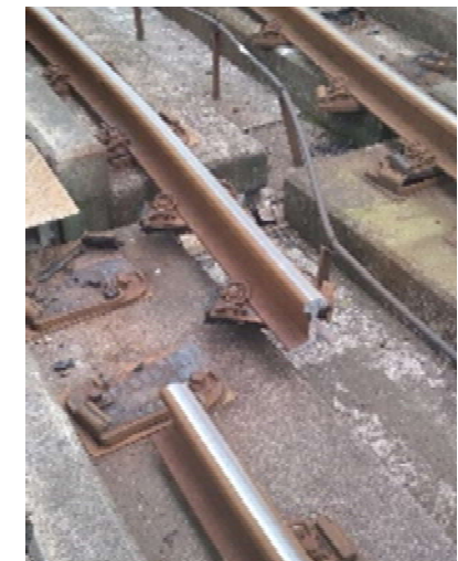
鋼軌變形斷裂
