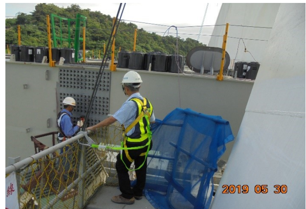
Fig. 11. The bolt tightening of steel truss frame under the first author’s supervision.
