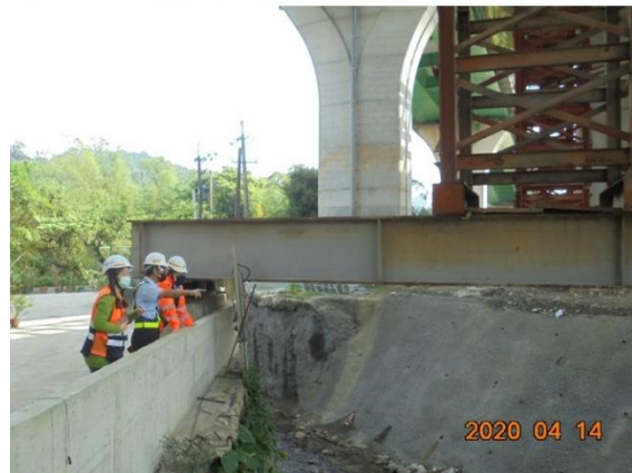
Figure 11: The inspection of the supporting beams by the corresponding author with the client engineers
