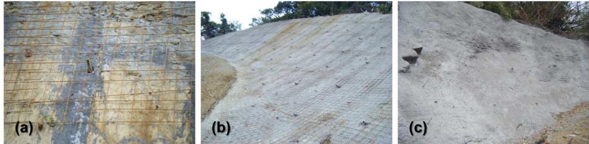
Figure 6 The appearances of the shotcrete structure slopes in different stages: (a) installation of wire meshes and SN anchors, (b) first layer spraying of shotcrete, and (c) finish of final shotcrete slope surface
