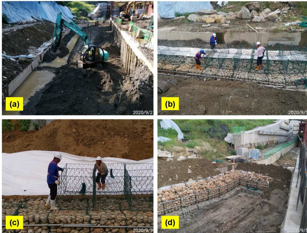
Figure 9 The work processes of the gabion structure: (a) excavation for the pond, (b)&(c) installation for wire mesh boxes, and (d) filling of the gravels
